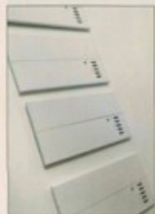
The house's main lighting control panels — even when hidden from view, as these are in a closet — are carefully aligned.
